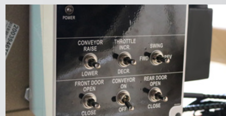
Manual override switch controls
